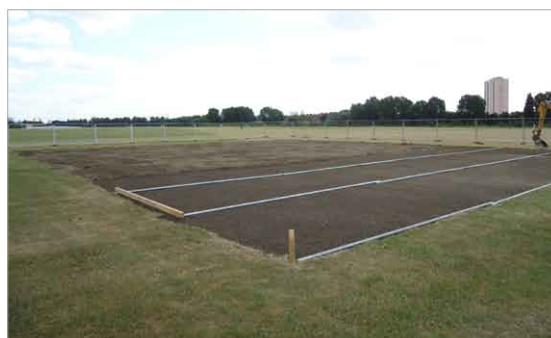
Precise placement and consolidation of cricket loam is crucial to the success of cricket square construction
